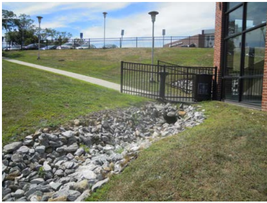
Figure 1: UNH's hillside riprap, installed after the 2012 campus flooding event in Kaplan Hall.
